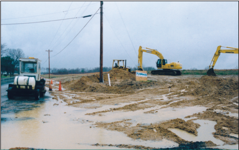
No Erosion Control at Construction Site
