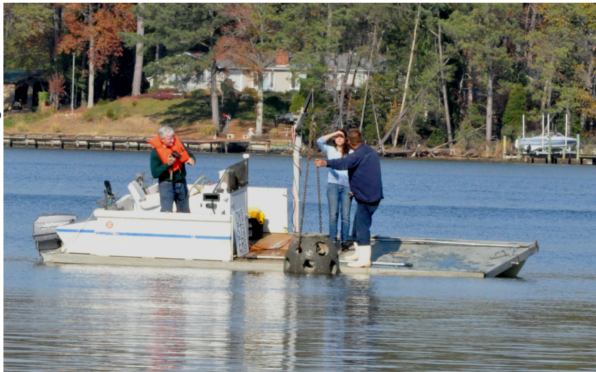
Representatives from the three project partners deploy the first reef ball onto the site of the St. Mary's River Reef Project. The three-dimensional structures installed in the river mimic historic oyster reefs, which can host four times the number of oysters than can be found on thriving flat oyster bars. Photo by Carrie Munn.
