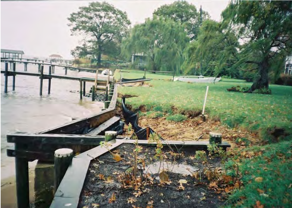
Fig. 31. Failed bulkhead with erosion behind structure. (Photo: Maryland Department of Natural Resources)
