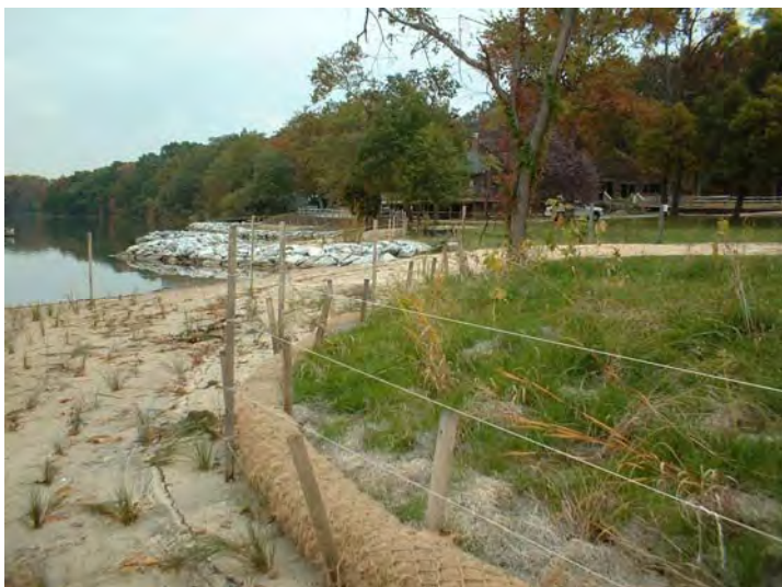
Fig. 8. Fiber logs provide temporary stabilization for a newly created marsh. A fence prevents waterfowl from eating young plants. (photo: Department of Natural Resources)
