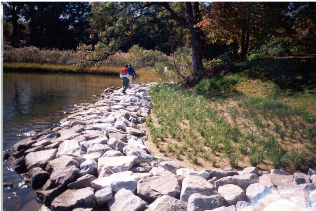
Fig. 23. Failed marsh establishment project. (photo: Maryland Department of the Environment)
