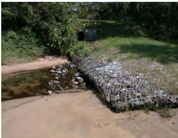
Fig. 29. Failed gabion baskets. Photo: Maryland Department of Natural Resources
