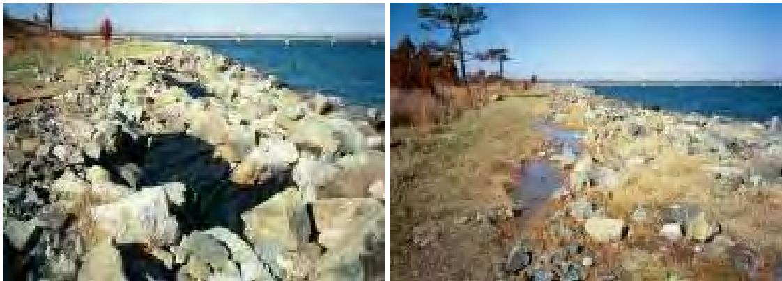
Figs 26 and 27. Failed revetments showing open area where rocks have shifted. (Photos: Maryland Department of Natural Resources)
