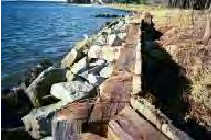
Fig. 30. Collapsing bulkhead with additional riprap. (Photo: Maryland Department of Natural Resources)
