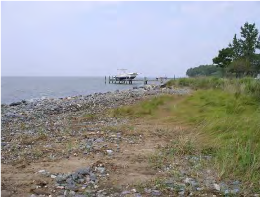
Fig. 11. Improper Fill. Photo: Team SWAMP, University of Maryland)
