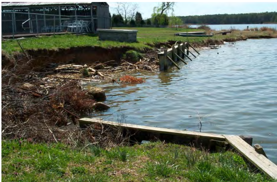
Fig. 32. Catastrophic bulkhead failure, resulting in need to replace entire structure with different stabilization practice. (Photo: Maryland Department of the Environment)
