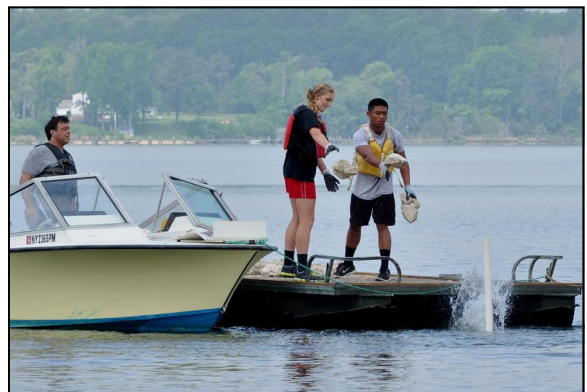
NHS students build concrete rubble mound as volunteer captain Charlie Sirico looks on. (May)
